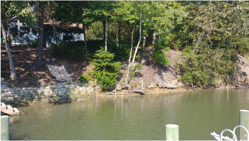
Shoreline. Envirolok Bags are shown on the right and on the left is the eroding shoreline where the Envirolok Bags are planned to be installed to the property line.
