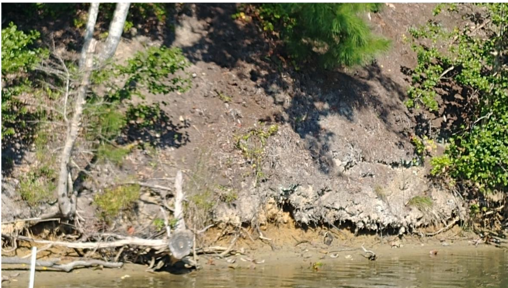
Close-up of the bank erosion on the shoreline. This is where the Envirolok Bags are planned to be installed.
