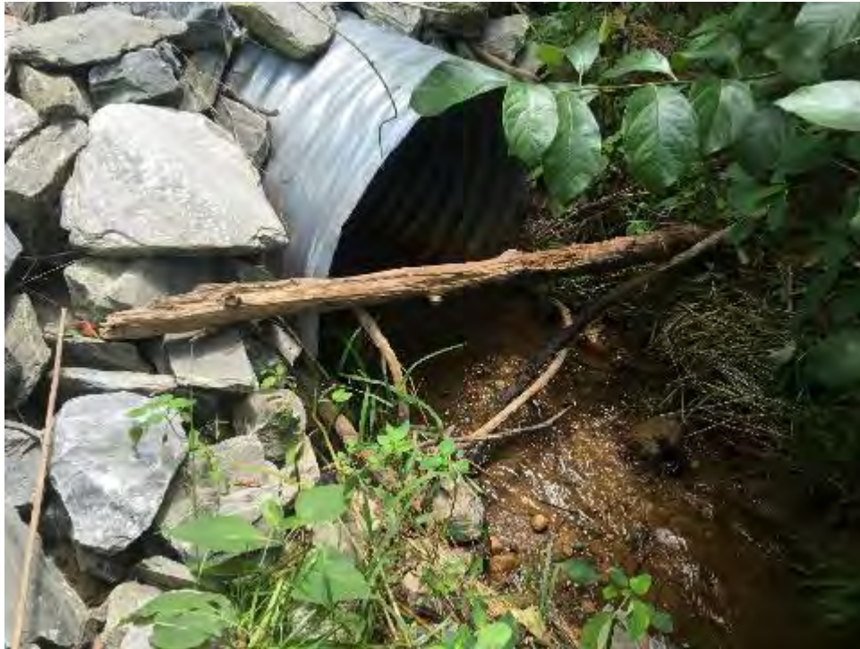
Debris at inlet
