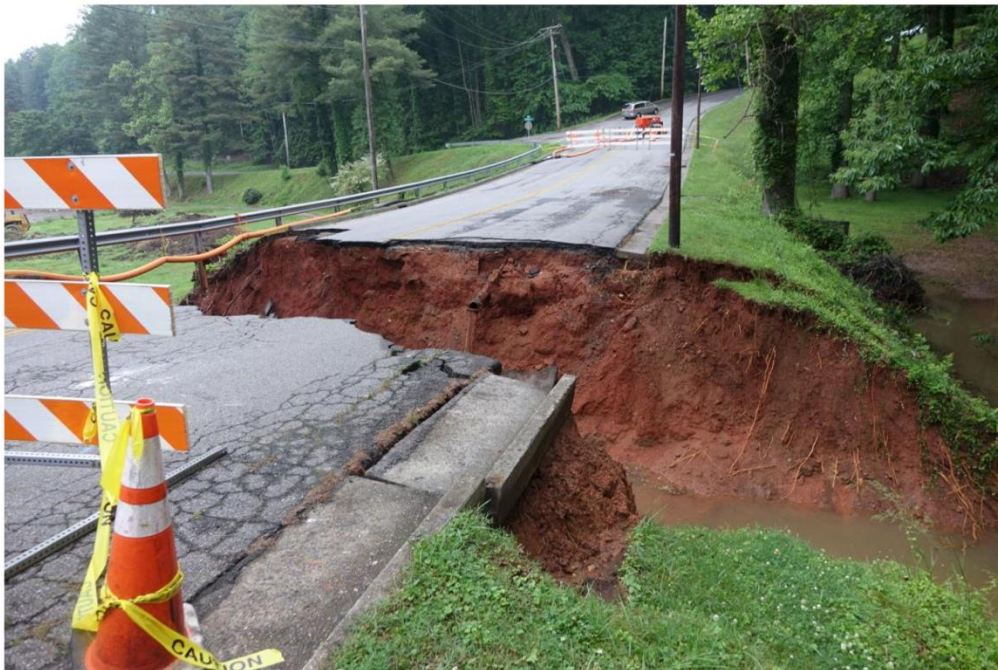
May 2018: Cherokee Trail collapsed after a heavy flooding
