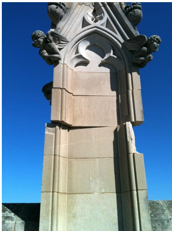
Figure 26: Earthquake Damage to Washington National Cathedral in Washington, D.C. After the 2011 Earthquake 77
