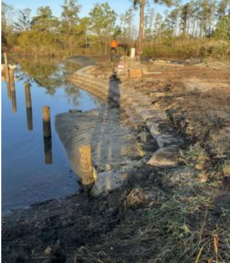
Figure 7 (above): Recently permitted and constructed project utilizing geotubes filled with dredged material in Gloucester. The tube has been covered with sediment and tidal marsh grasses have been planted atop the tube as part of a living shoreline.
