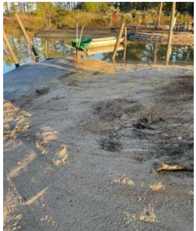
Figure 8 (right): Recently permitted and constructed project utilizing geotubes filled with dredged material in Gloucester. The picture shows the tube as it is being covered with sediment. Grass has since been planted atop the tube as part of a living shoreline.
