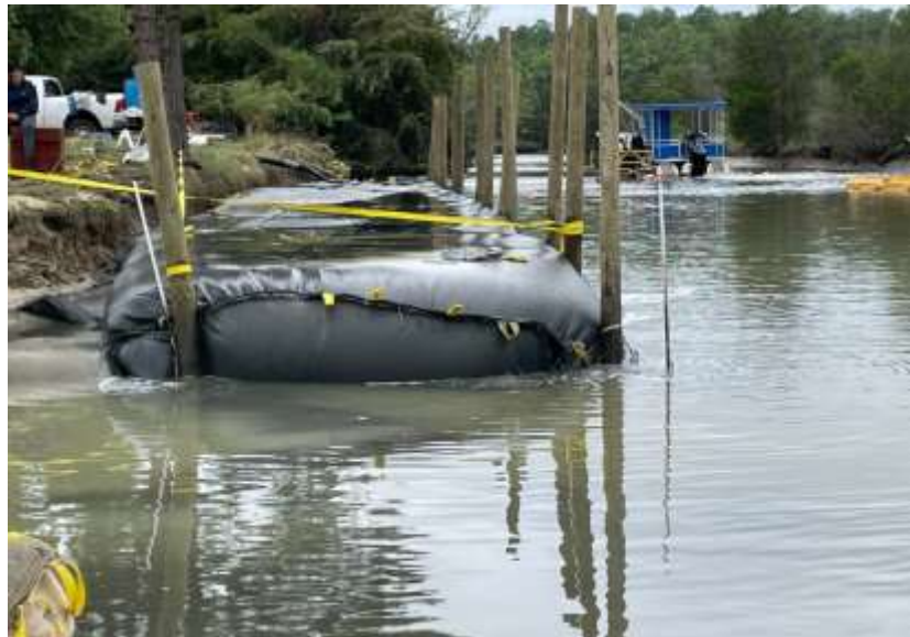
Figure 6: Recently permitted and constructed project utilizing geotubes filled with dredged material in Gloucester. The tube has been covered with sand and grass and will function as a docking area at a public boat landing.
