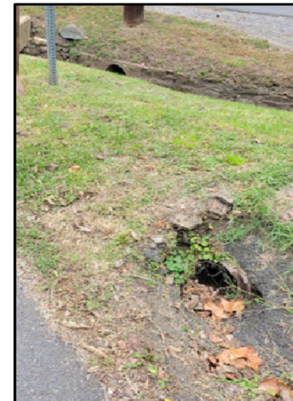
PHOTO 5 INADEQUATE STORMWATER INFRASTRUCTURE
