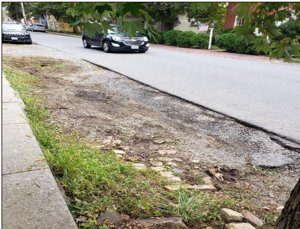
Photo 6. Lack of Stormwater Drainage Infrastructure on Main Street / Erosion.
