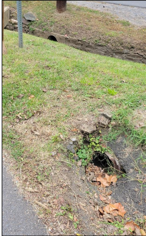
Photo 11. Inadequate Stormwater Drainage Infrastructure
