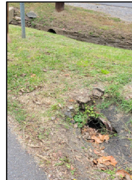
PHOTO 5 INADEQUATE STORMWATER INFRASTRUCTURE
