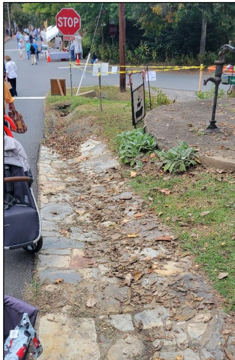
Photo 10. Inadequate Stormwater Drainage Infrastructure
