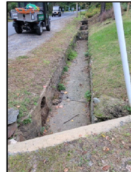
PHOTO 6 INADEQUATE STORMWATER INFRASTRUCTURE
