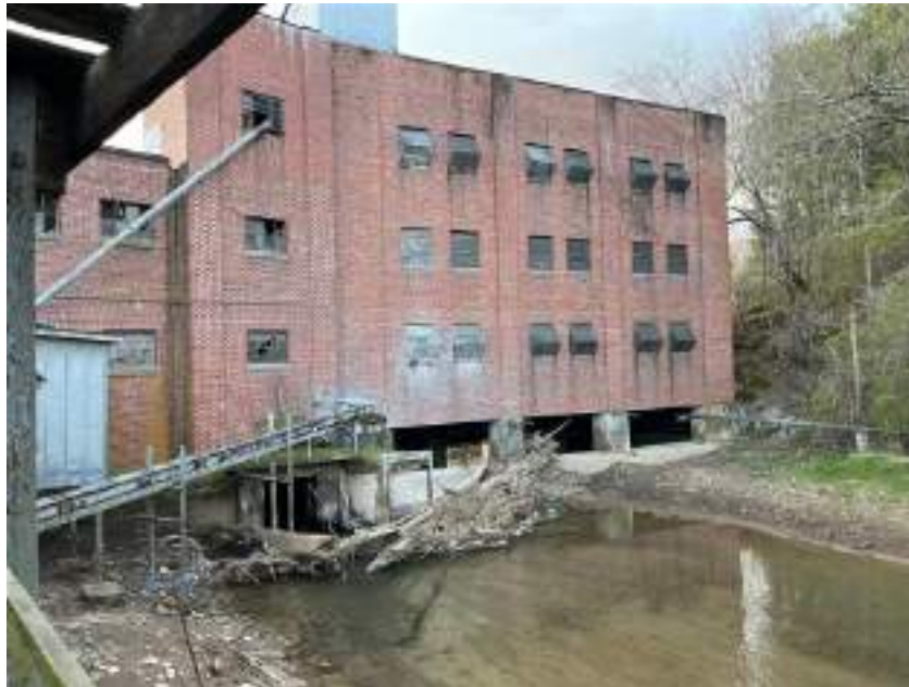
Figure 76: Example of debris captured on dam in North Tazewell
