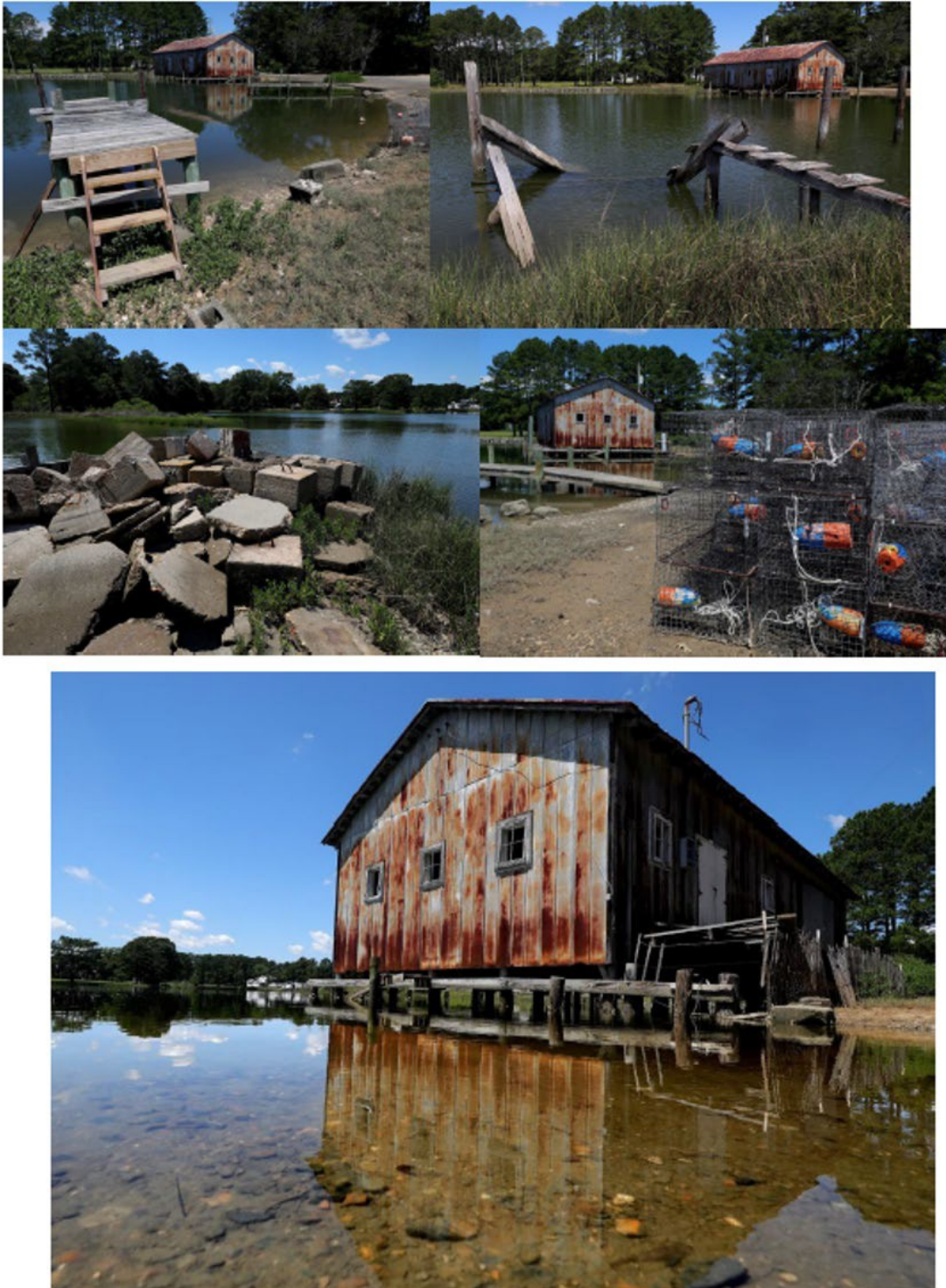
The images of site damages are all a result of flooding and coastal weather events.
