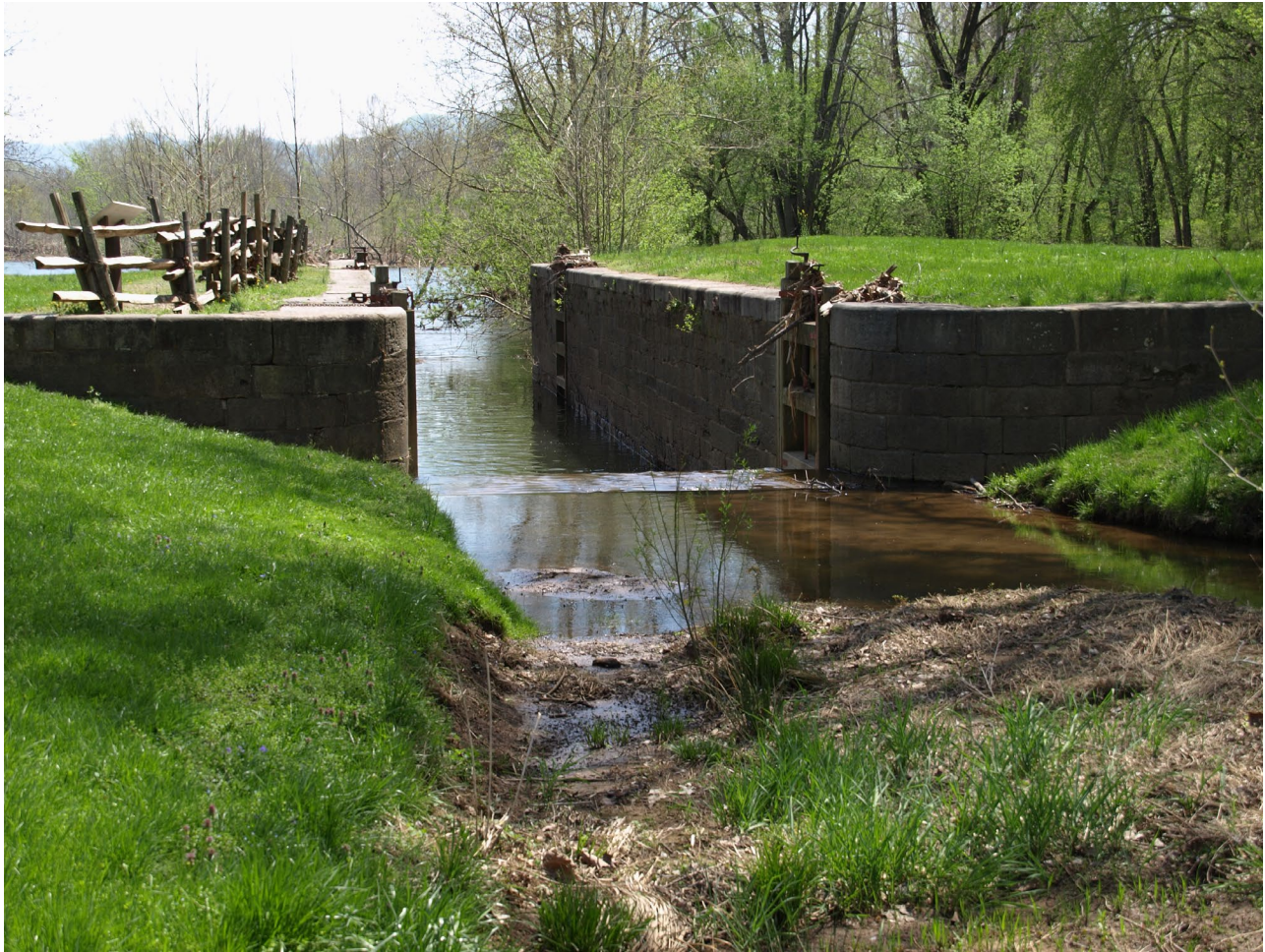
Figure 28 Battery Creek Lock on the James River at the Blue Ridge Parkway, photo by Gary Kappesser
