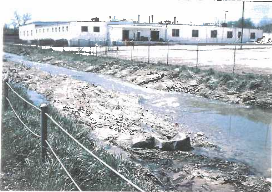
Indian Gap Run after April 1992 flood. Reeves Brothers Plant in background.
