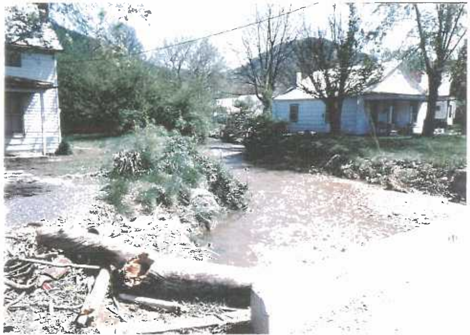
Debris and sediment blocking street culvert near confluence of Noels and Indian Gap Runs after April 1992 flooding.
