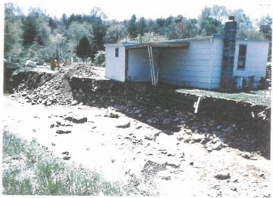
Scouring of stream channel on Pedlar Gap Run after April 1992 flooding.
