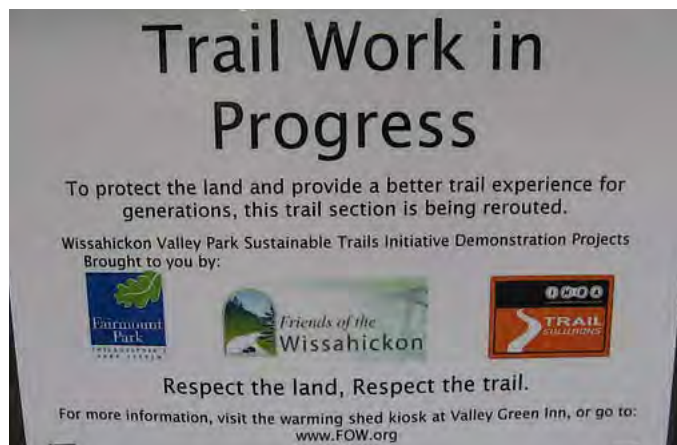
Trail closure and re-routing sign. Courtesy of IMBA/Rich Edwards.
