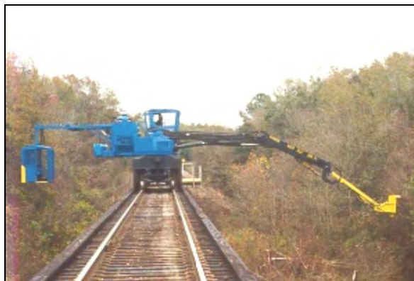
Source: AREMA, IPRE Seminar, Module 7: Track and ROW Maintenance PowerPoint, Chicago, Sept. 2005
