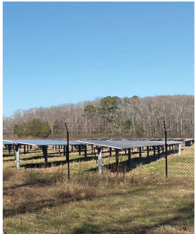
Gloucester Solar Electric Power Plant - Located off Rte. 14, the first Board approved utility-scale solar energy facility within the County.
