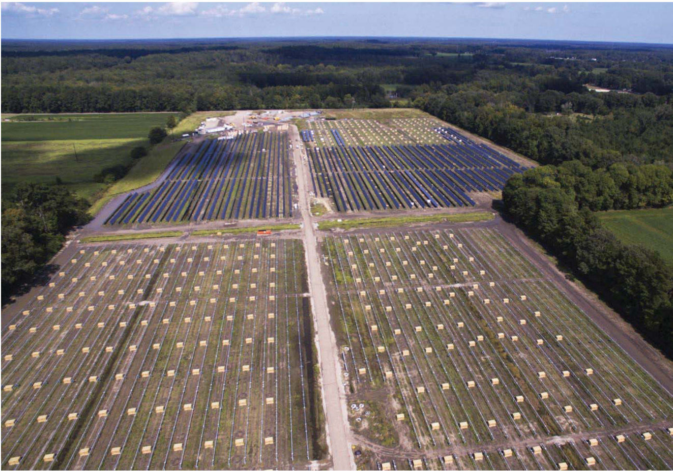
Aerial during construction of Gloucester Solar Electric Power Plant - Located off Rte. 14, the first Board approved utility-scale solar energy facility within the County. Source: SUKUT Construction.
