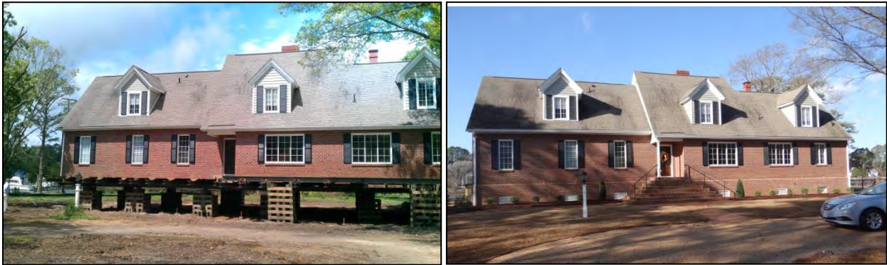
Figure 81: Photos of an elevated home in Moon, Va during (left) and after (right) (Mathews County, 2015).
