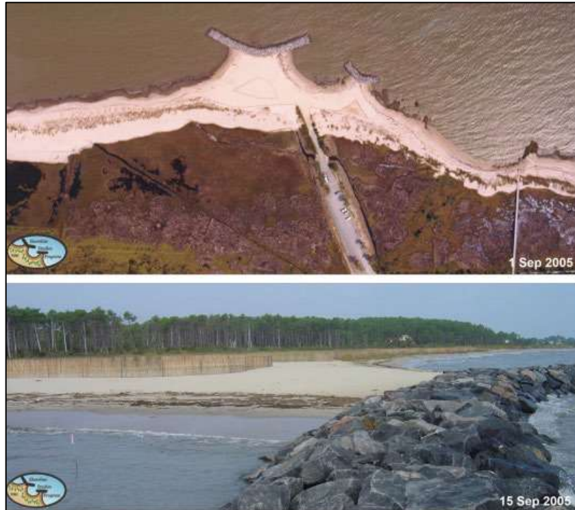
Figure 11 - Aerial photo (top) and ground photo (bottom) taken at Haven Beach after breakwater and beach fill installation in 2005.
