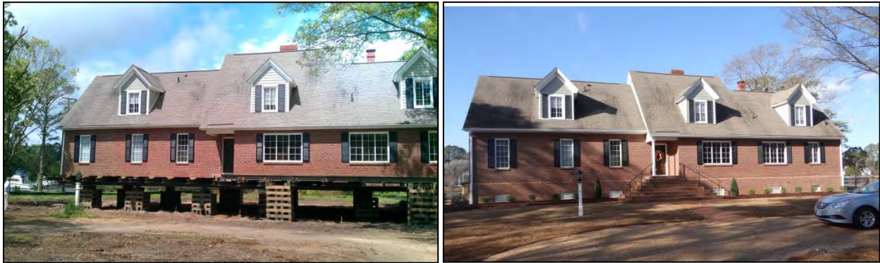
Figure 81: Photos of an elevated home in Moon, Va during (left) and after (right) (Mathews County, 2015).
